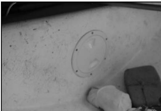
APPROVED CHANGE #30 - INSPECTION PORT
